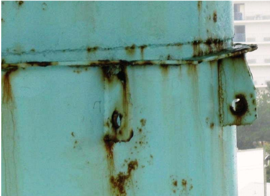
Photo #8 Corrosion on the upper riser pipe.
