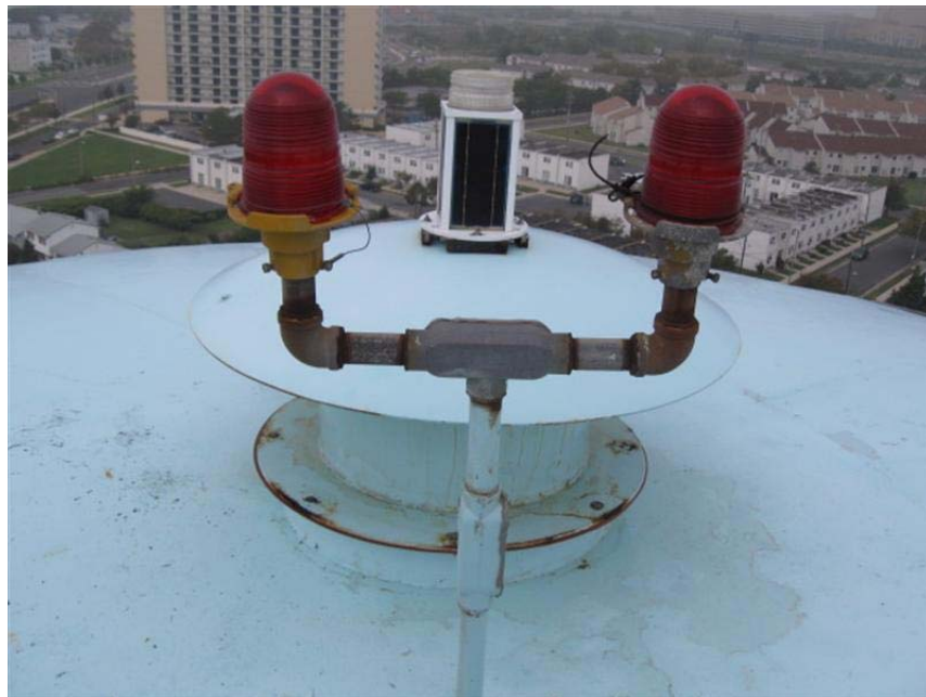
Photo #24 Aviation warning like on the roof is not functioning. New battery-operated aviation flight has been attached to the roof vent. Photo also shows center roof vent.
