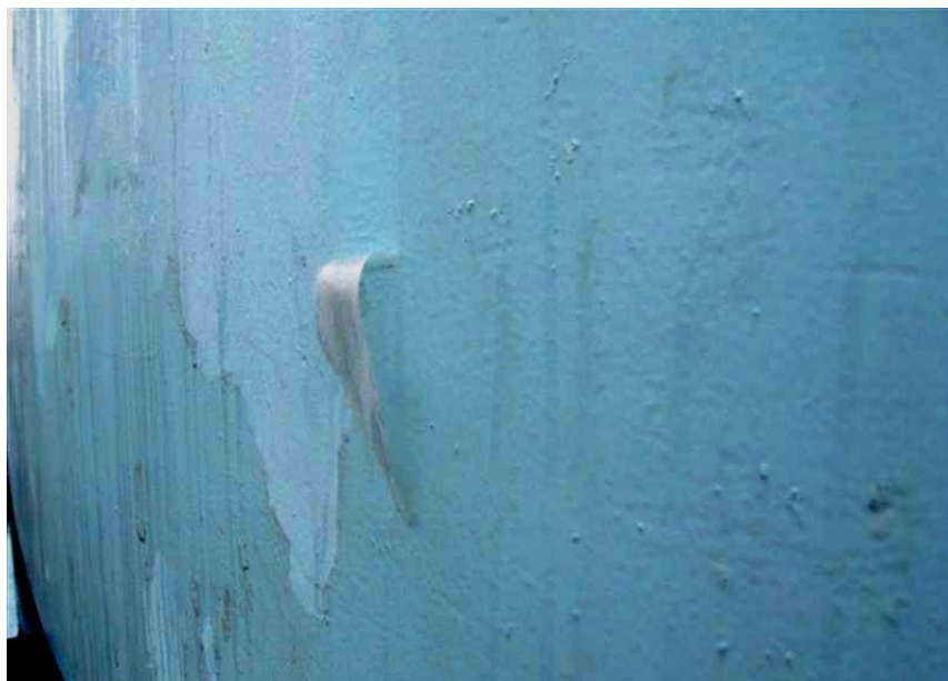
Photo #2 Coatings on tank riser pipe are in good to fair condition. Chalking and minor mildew growth is evident, along with delaminating clear coat.
