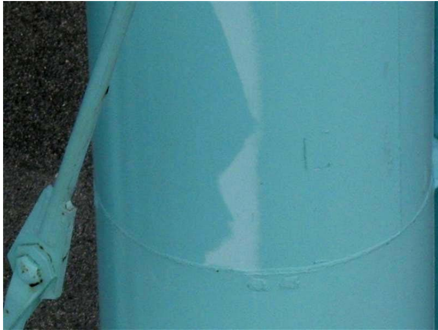
Photo #1 Coatings on exterior legs are in good condition. Clear coat finish is beginning to delaminate.
