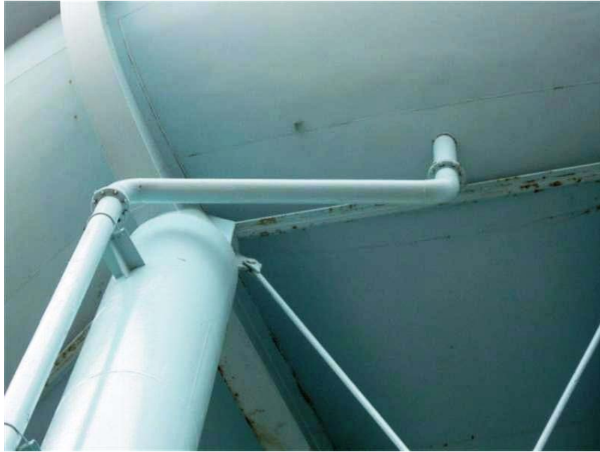
Photo #29 Overflow pipe is secured to the leg and is in good condition
