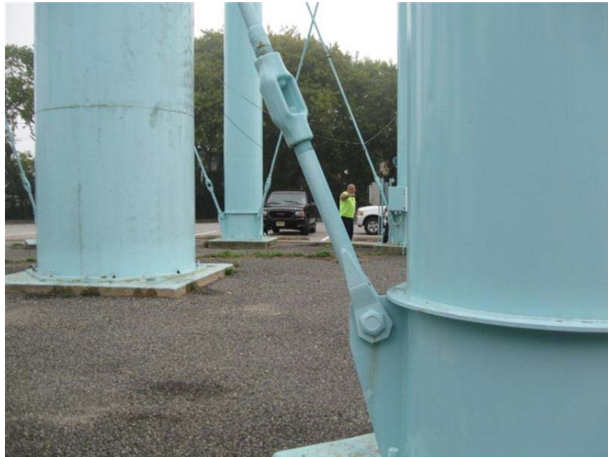
Photo #36 Wind rod yokes and turnbuckles are in tight and in good condition.
