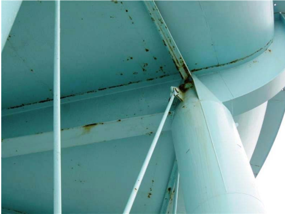
Photo #5 Corrosion and mildew growth on underside of tank bowl and on the structural beams.
