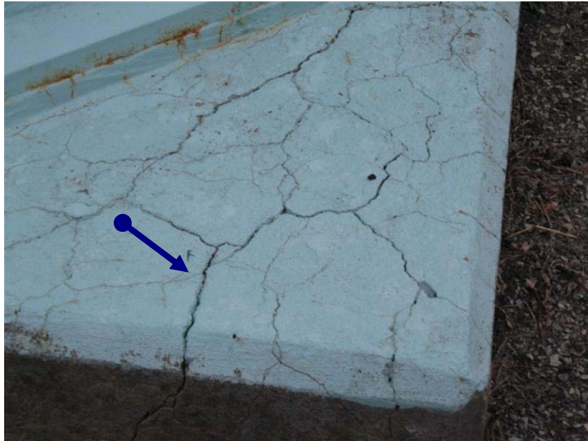
Photo #32 Cracks should be filled and sealed to prevent the intrusion of water and possible freeze-thaw damage to the foundation.
