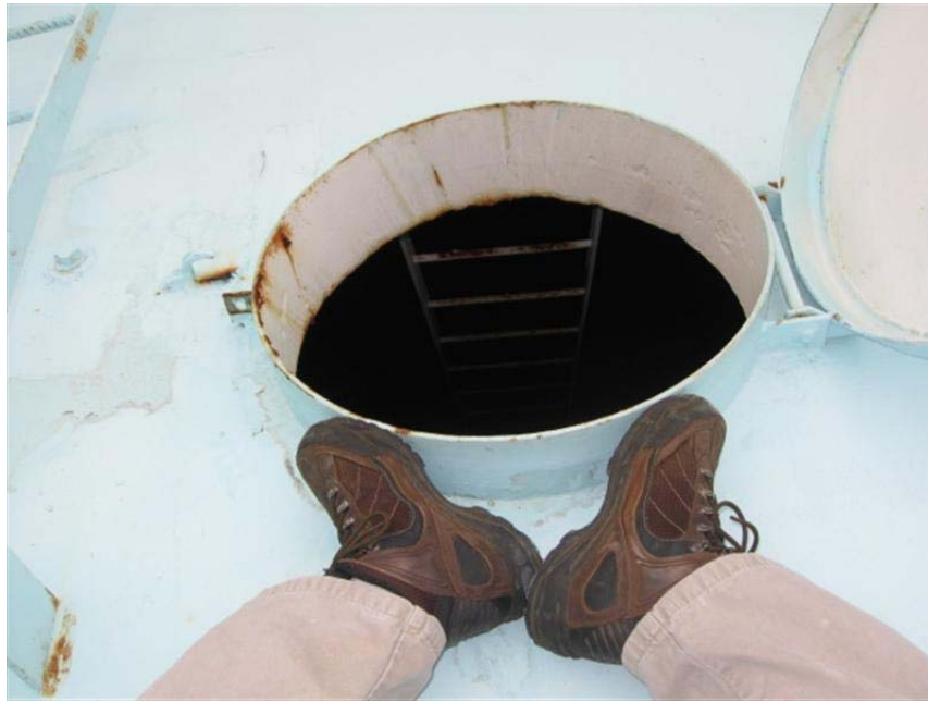
Photo #27 24" round roof access hatch. Roof hatch cover overlaps curb to prevent contaminated rainwater from entering the water chamber.
