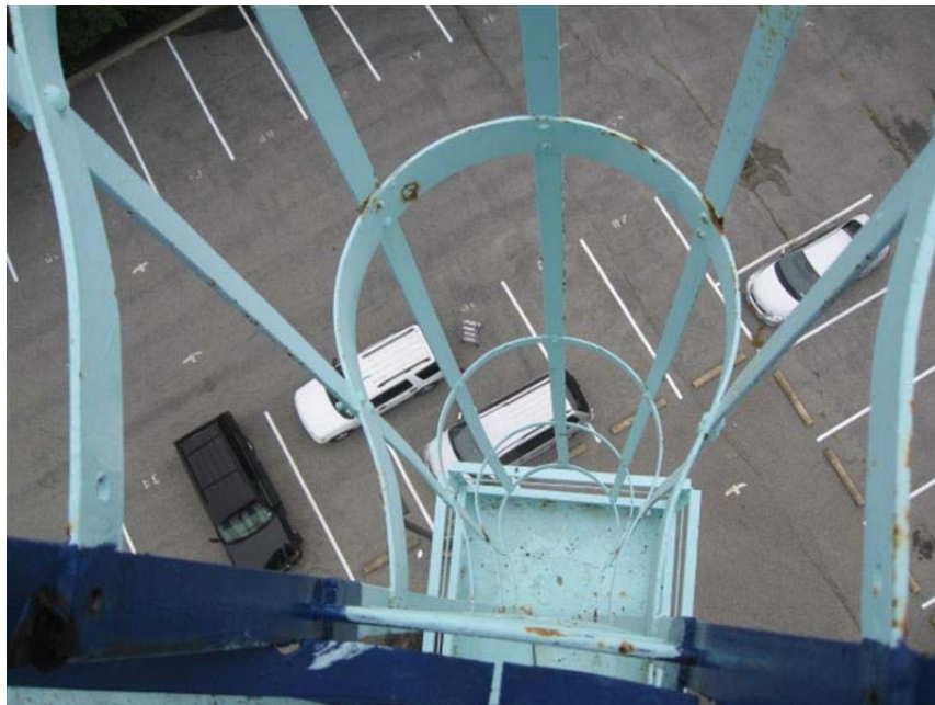
Photo #20 Second tier access ladder does not contain a suitable safety climb device.
