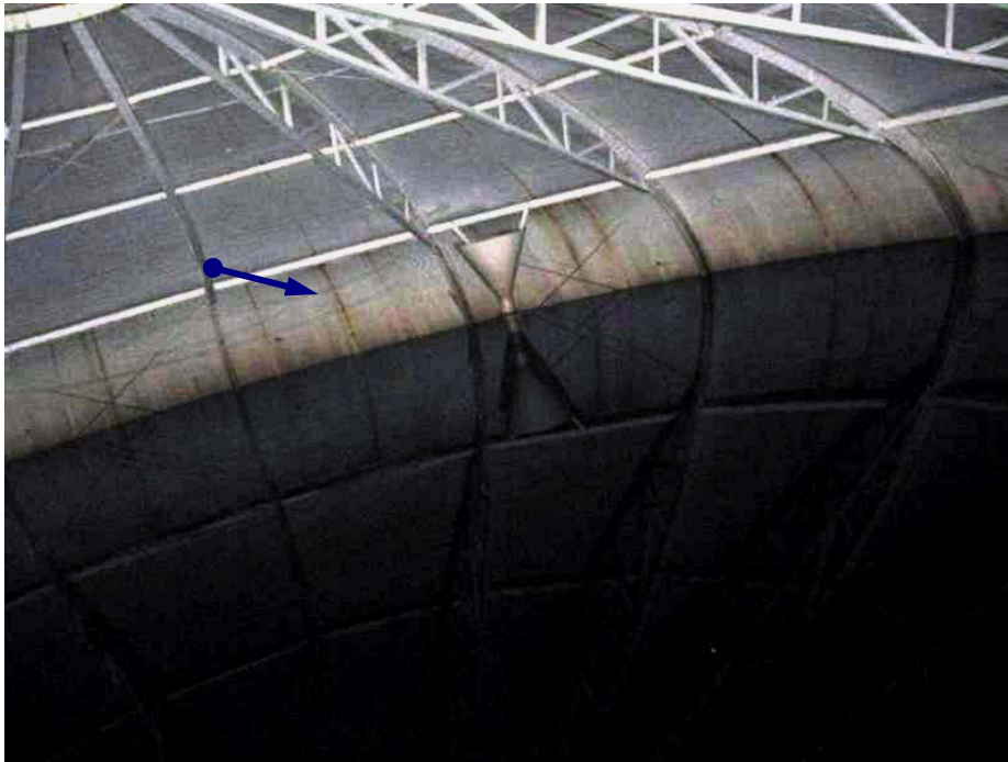
Photo #13 Coatings on the interior are in good condition with some minor corrosion and organic staining on the sidewalls and roof.
