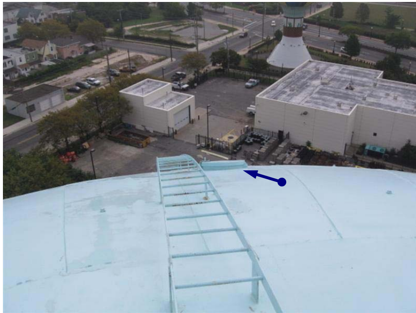
Photo #28 Roof access hatch meets current standards and was not locked at the time of the inspection.
