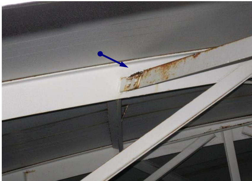
Photo #14 Coatings on interior roof and above the high water level are in fair condition. There is active corrosion and delamination on areas on structural beam edges.
