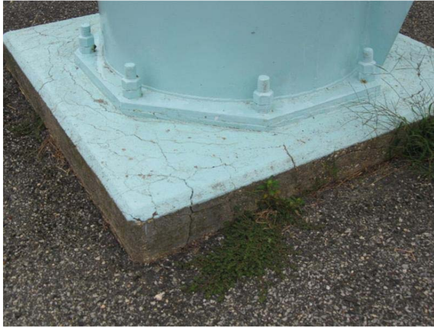
Photo #31 Foundation piers are in good to fair condition. There are moderate levels of cracking and spalling on several of the foundation piers.
