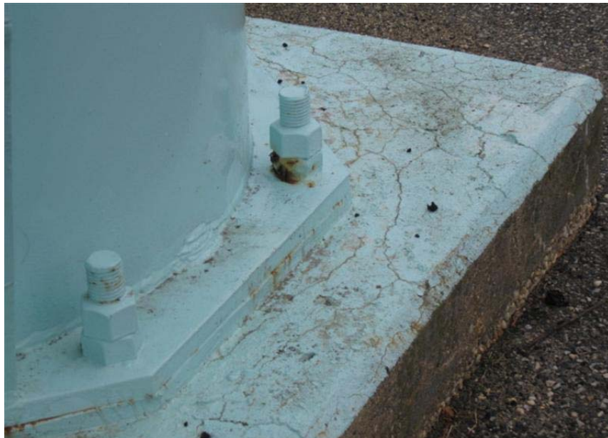
Photo #38 Anchor bolts and nuts are in generally good condition with only moderate levels of corrosion on several of the nuts.
