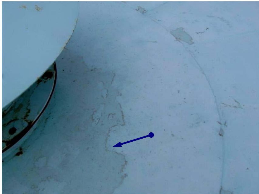
Photo #12 Coatings on roof are thinning and clear coat finish is wearing and delaminating.
