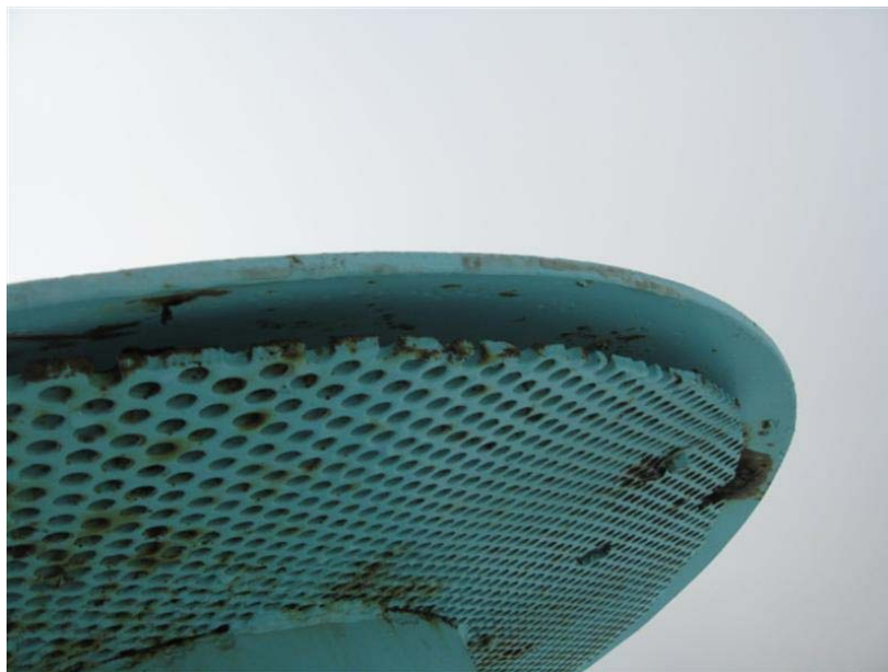
Photo #26 Roof vent does not meet current standards and should be replaced with a modern aluminum frost proof that system to prevent insects and birds from entering the water chamber.
