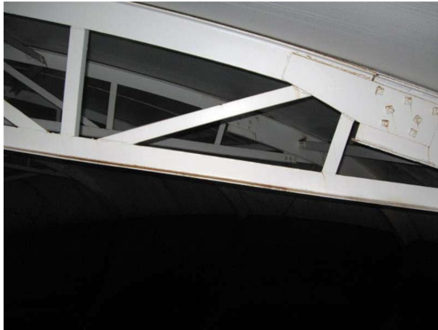
Photo #16 Coatings on roof structure and panels are in generally good condition.
