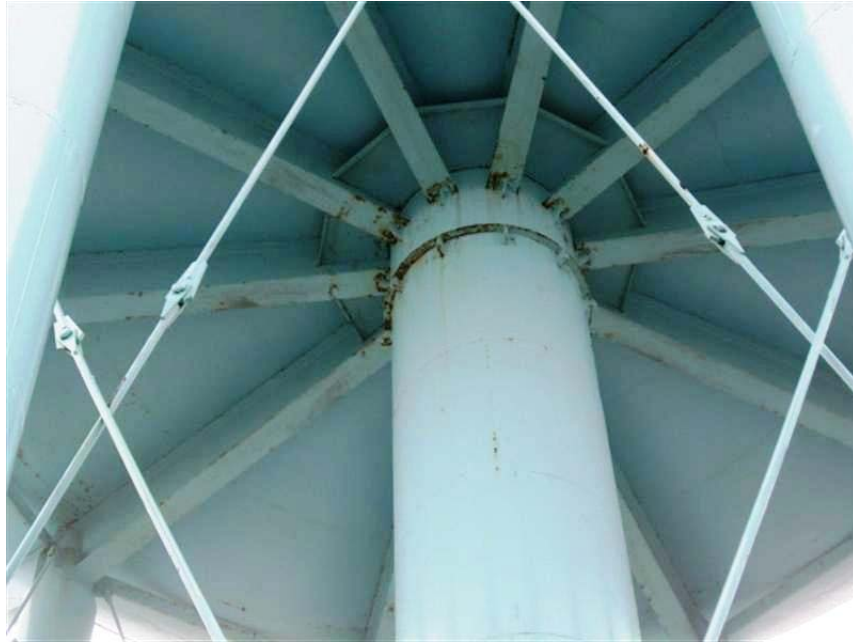
Photo #7 Chalking of coating, and minor to moderate levels of corrosion on underside of tank bowl.
