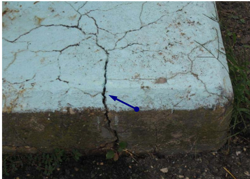
Photo #34 Cracking and spalling of concrete foundation piers
