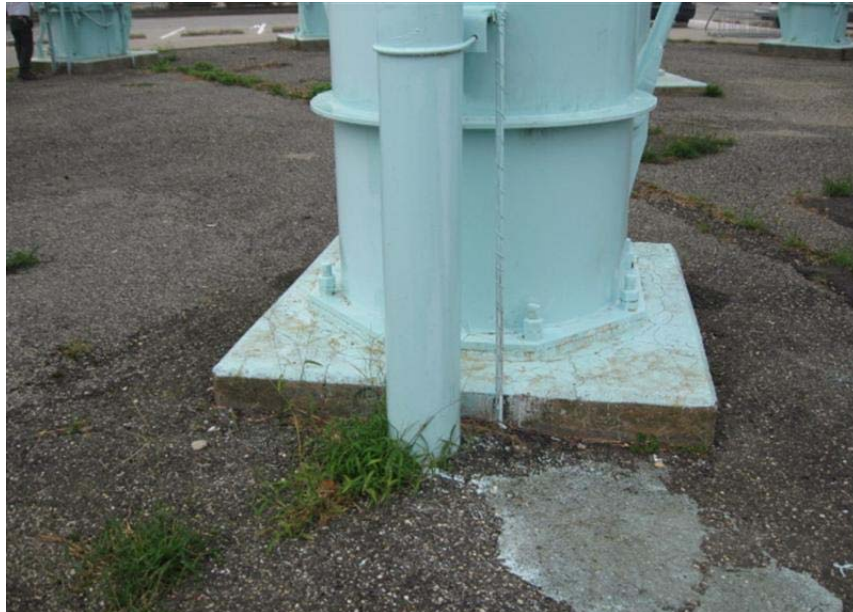
Photo #30 Overflow terminates below grade and likely has an outlet in the adjacent street. Further investigation should be done to ensure a proper vent screen is in place to prevent vermin from entering the water chamber.
