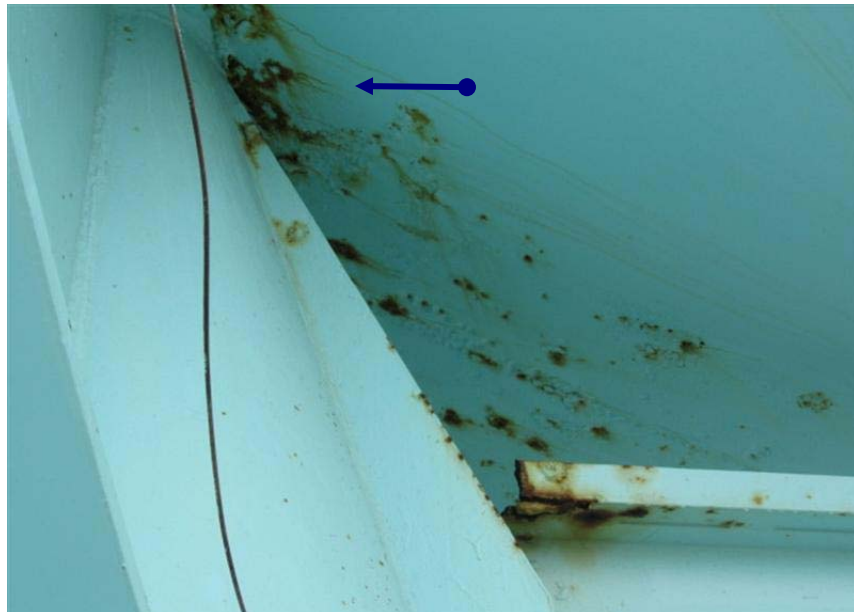
Photo #6 Corrosion and mildew growth on the underside of tank.
