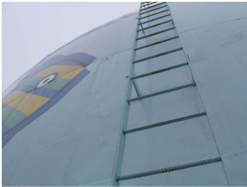
Photo #21 Upper sidewall ladder is in good condition but does not contain a suitable safety climb device.
