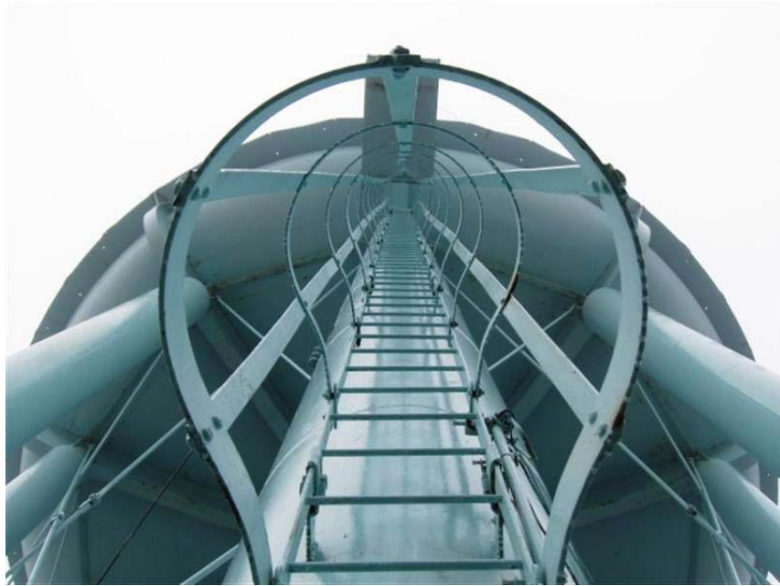
Photo #17 Main access ladder is in good condition, but does not contain a suitable safety climb device or a tamperproof ladder gate.
