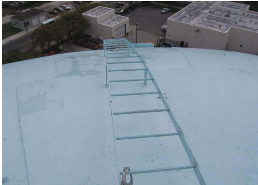
Photo #22 Dome roof ladder is secure and in good condition, but does not contain a safety climb device.
