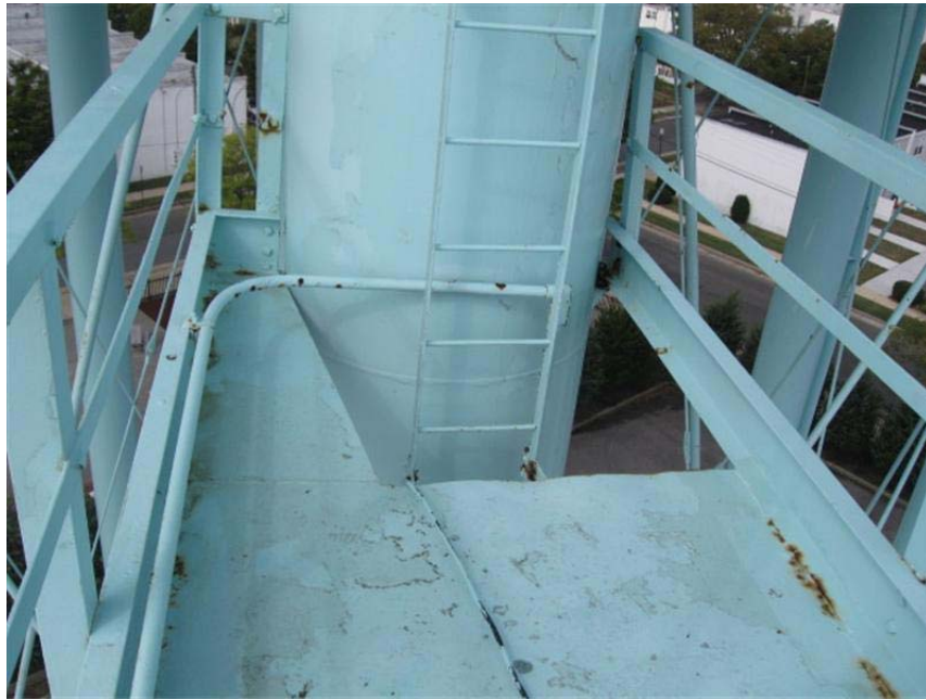
Photo #19 Areas of moderate corrosion on ladder balcony. Clear coat finish his delaminating on balcony floor.
